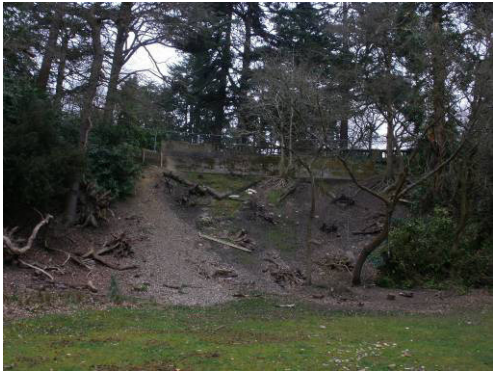
Photo 14 – Unstable wall and temporary fence (A8)
