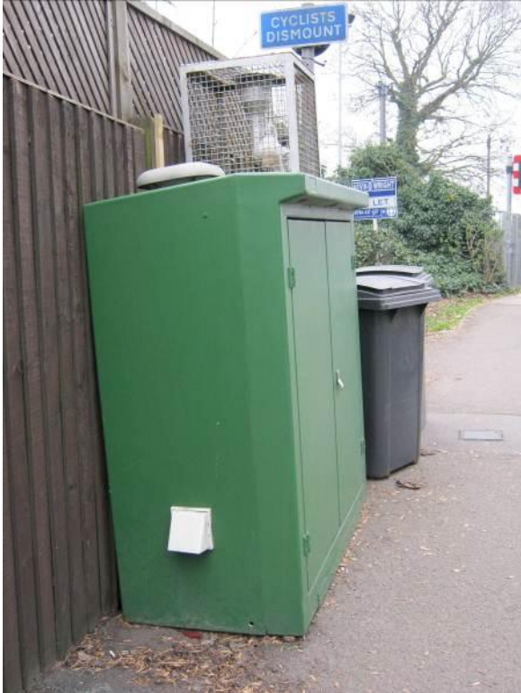
Figure 2-2 Site Photos of Automatic Monitoring Station in Egham
