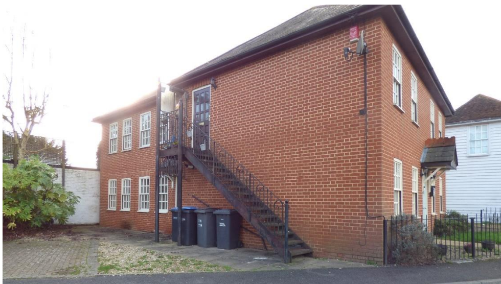
Figure 49: The staircase and satellite dish on the side of The Carriages are unwelcome features within the Conservation Area.
