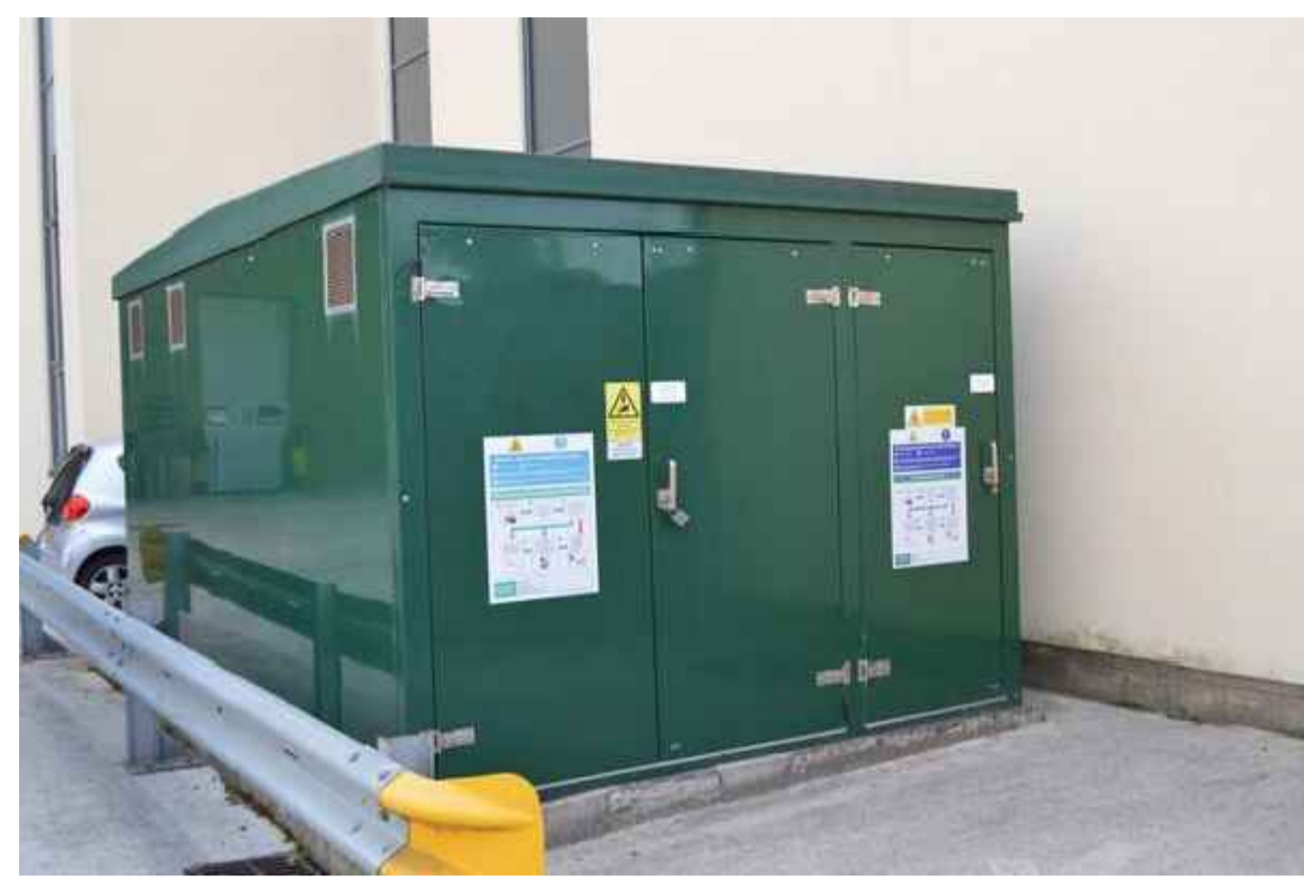
Substation Typical glass reinforced plastic housed substation to meet energy and power distributor's specification. Size: 3.0m x 3.0m x 2.5m high, with double-door aperture of 2.7m x 2.1m high. Colour: 18 B 25 (Merlin Grey or Green) to meet standard approved colours defined by energy and power distributor in accordance with BS 4800: 2011.
