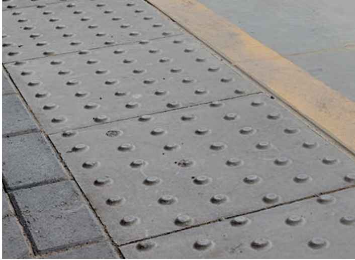
Tactile blister paving demarcating changes in level
