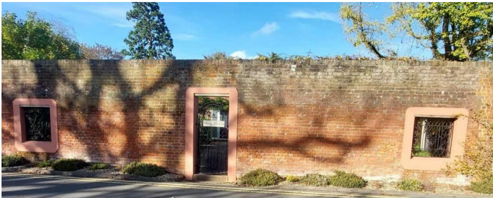
Figure 63: Inappropriate holes inserted into the red brick wall along Coldharbour Lane, close to the junction with Ten Acre Lane.
