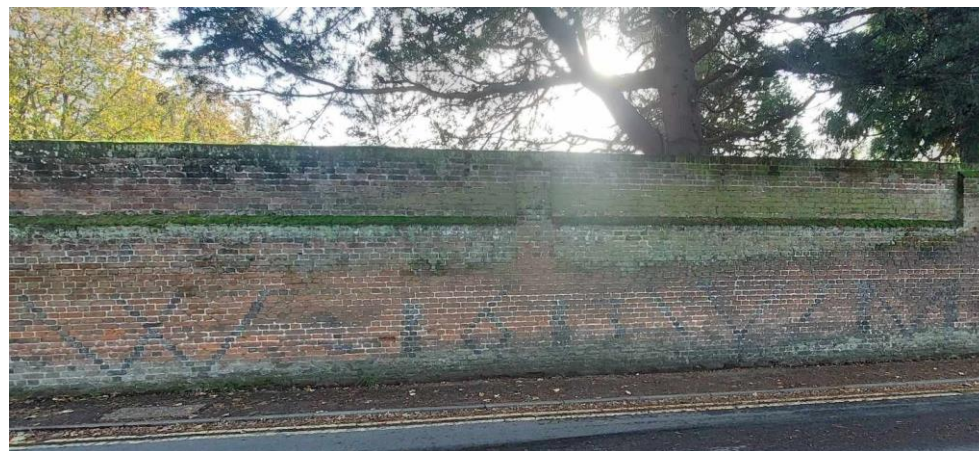
Figure 7: Diaper brickwork in the boundary wall on the south of Coldharbour Lane, spelling W 1613 W M.
