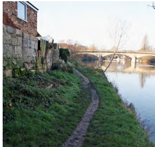
The narrow path and retaining wall in disrepair at the eastern end of the Thames Path
