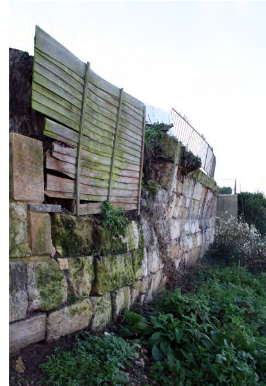
Bulging boundary wall along the Thames Path
