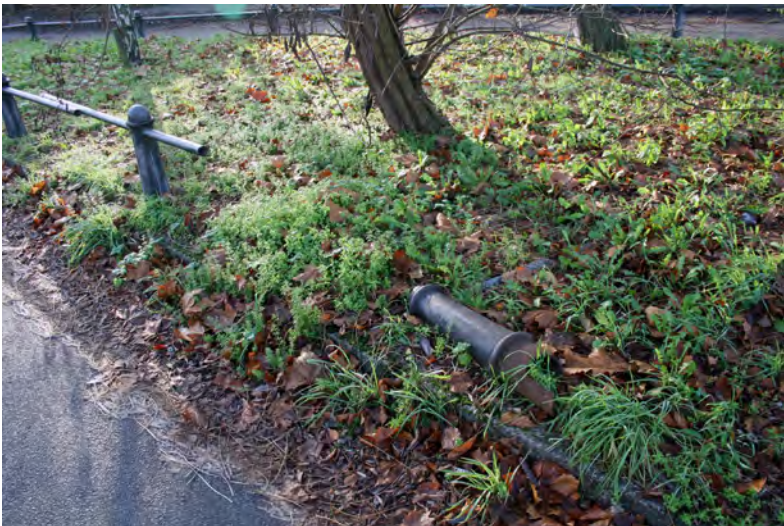
Broken railings and posts around the triangular green at the western end of The Hythe
