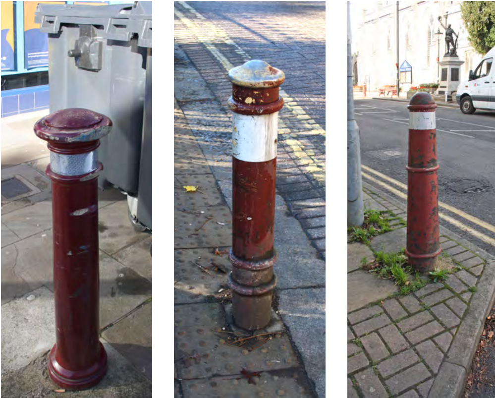
Bollards in Guildford Street, there are a variety of styles and many are in a poor state of repair
