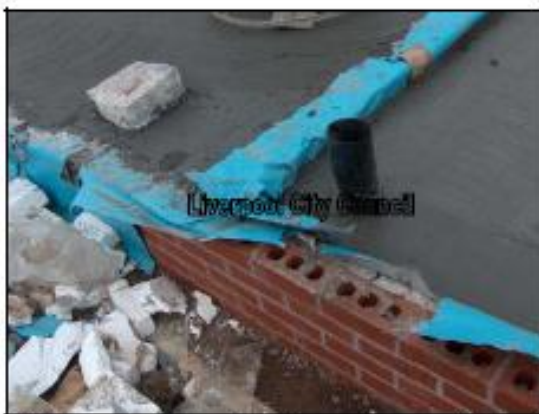
Jointing not sealed and membranes torn, as visible after casting of slab.
